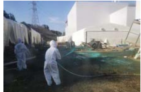
Workers spray adhesive synthetic resin over the ground at the Fukushima Daiichi nuclear power plant. Photo / AP
