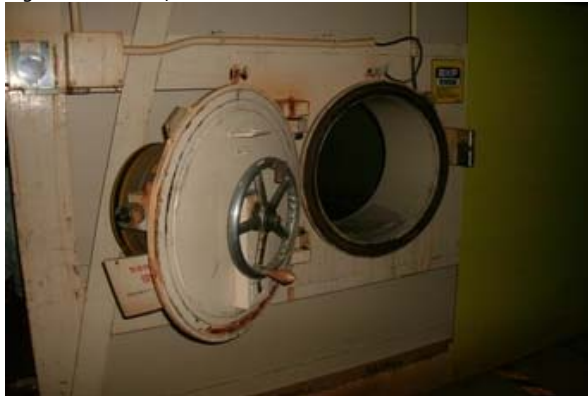
Fukushima Daiichi Unit 2 emergency exit; Image taken on 20 June as reactor building airlock opened
